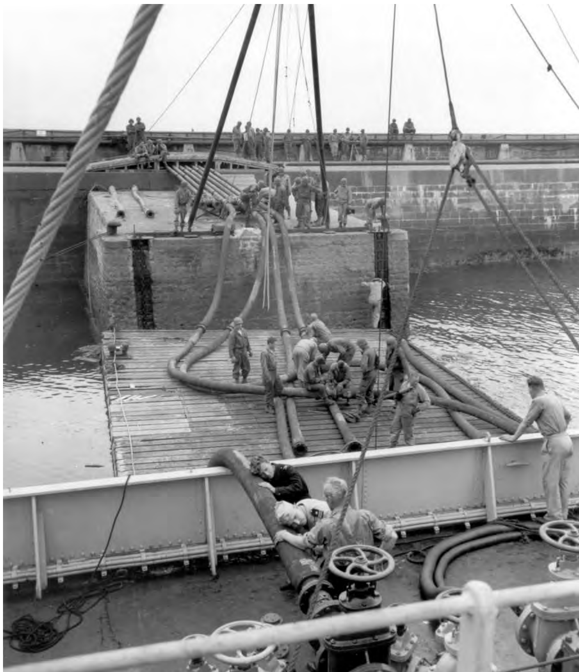
THE FIRST SHIP-TO-SHORE GASOLINE LINE, put in operation at Cherbourg. During the assault phase the Allied forces relied on canned gasoline, but by 3 July bulk supply was being introduced by ship-to-shore pipeline which brought in part of the large quantities of gasoline necessary to the Allied forces.
